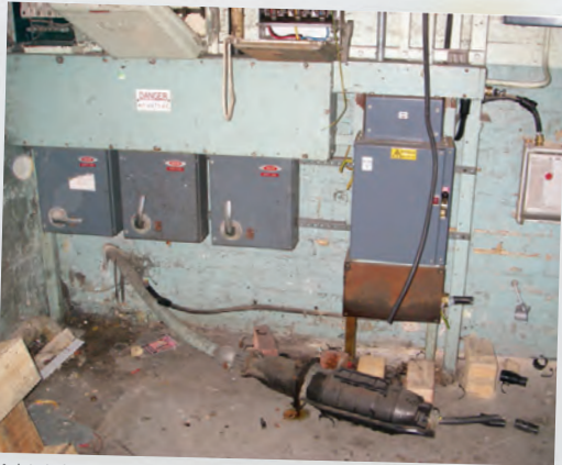
A high hazard electrical installation, with exposed conductors
